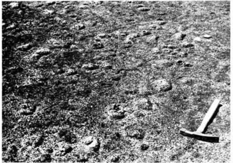
Figure 2: Blister zone. Blisters are hollow and some have collapsed.
