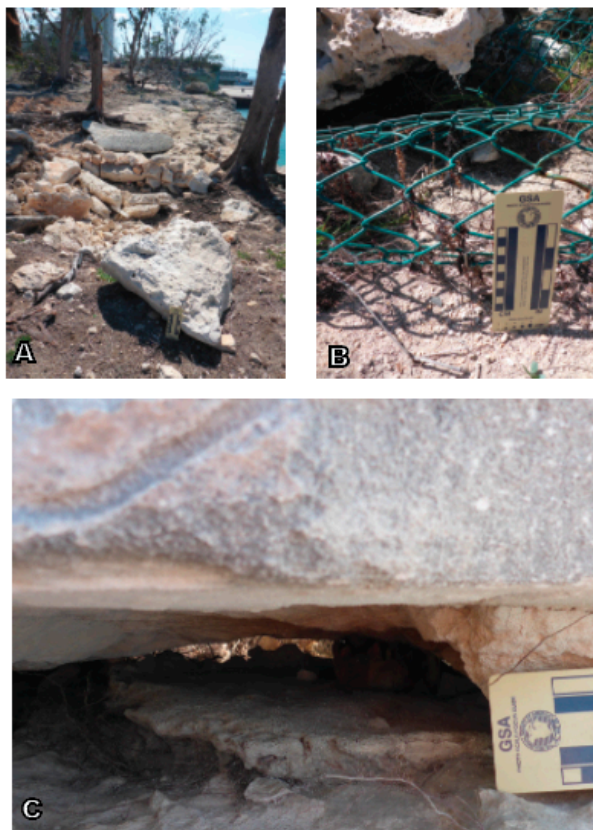
Figure 10: A) Small boulder apparently moved by rolling. B) Sea wrack entangled in the fallen fence. One of the boulders now resting atop the fence is visible at top of image. C) This is the very large slab of rock that previously formed the lintel over the Pirate Stairs. It has been shifted up, inland, and slightly to the west, and now rests directly atop the sheared off base of one of the metal fence posts (visible in the crevice). This slab is visible in Figure 8 A, as it originally rested, and the corner of it is visible on the right edge of Figure 8 B, in its post Hurricane Matthew location.
