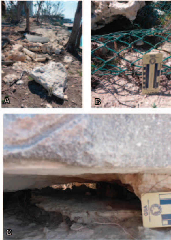
Figure 10: A) Small boulder apparently moved by rolling. B) Sea wrack entangled in the fallen fence. One of the boulders now resting atop the fence is visible at top of image. C) This is the very large slab of rock that previously formed the lintel over the Pirate Stairs. It has been shifted up, inland, and slightly to the west, and now rests directly atop the sheared off base of one of the metal fence posts (visible in the crevice). This slab is visible in Figure 8 A, as it originally rested, and the corner of it is visible on the right edge of Figure 8 B, in its post Hurricane Matthew location.
