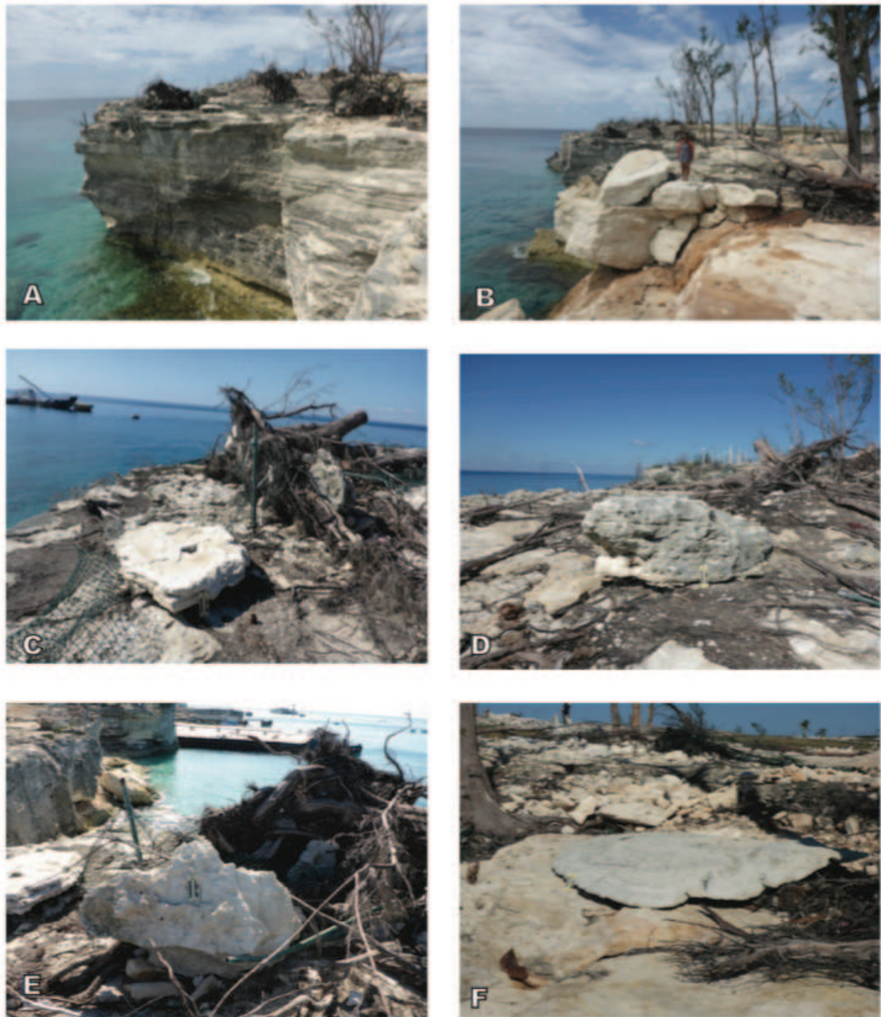
Figure 9: A) Cliff showing bedrock exposure immediately to the west of the Pirate Stairs. B) Very large boulder dislodged from top edge of approximately 6-m-high cliff, west of the Pirate Stairs (researcher for scale). Note the red caliche that lines the vertical and horizontal fracture surfaces. The unweathered surface of the cliff and boulders indicates recent collapse and movement. C) Boulder deposited on top of flattened fence. Also note uprooted Casuarinas Sp. D) Boulder moved inland and uprooted Casuarinas sp. E) Boulder deposited on top of remains of fence with uprooted tree and sea wrack. F) Waste concrete slab apparently lifted and slide inland. It's original location in approximately where the "F" is located on the image.
