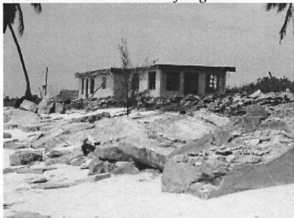
Figure 5. Broken seawall near Rocky Point.
