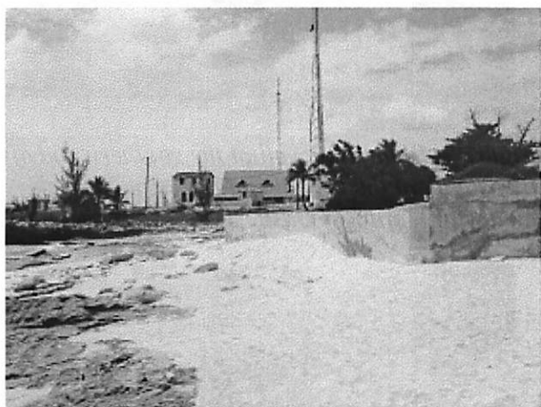
Figure 4. Seawall at Cockburn Town looking northward toward the radio towers and Catholic Church. Beachrock is in foreground.
