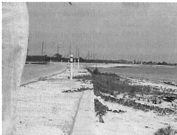
Figure 6. Seawall at Fernandez Bay looking south. Queens' Highway is on left. White poles demarcate the wall edge.
