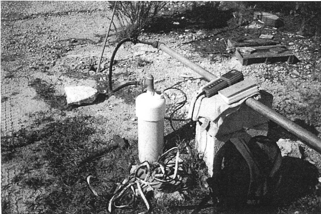
Figure 7: Typical well head at the Airport Well Field.
